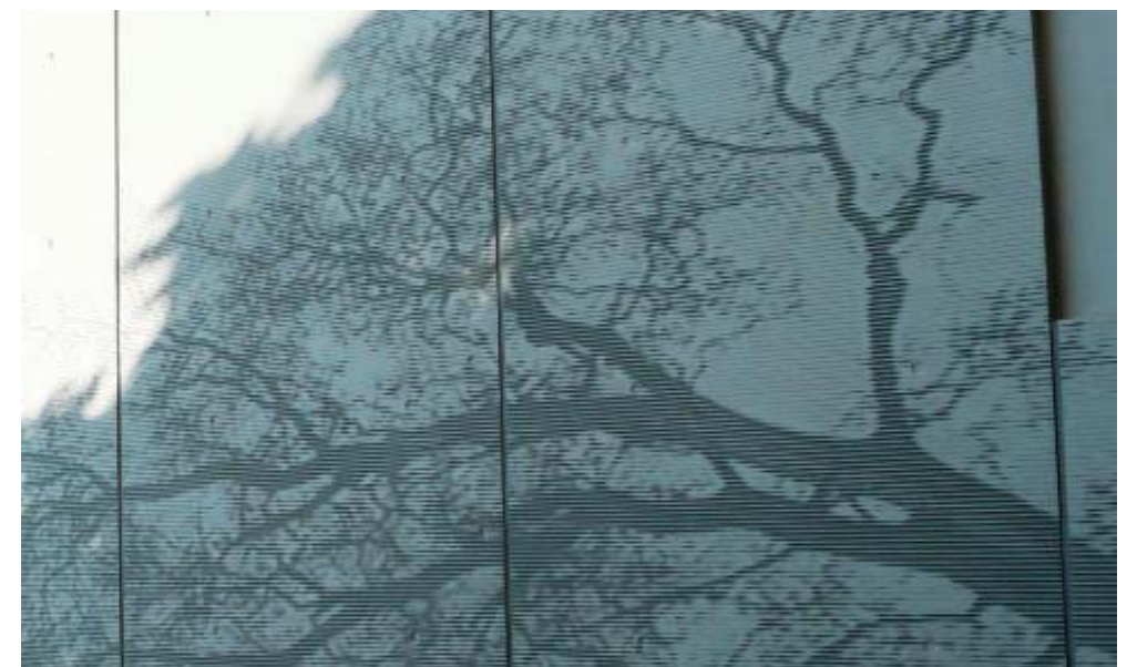
Concrete Cladding (including etched lettering) Reckli or similar Concrete is used to define the edges of the King Street Link, the boundary to the Interchange building, and the rail platform.
